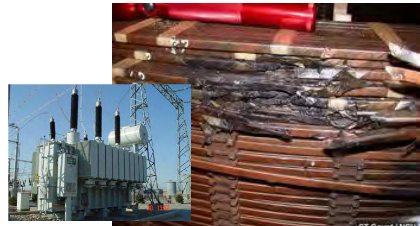
Damage to high voltage transformer, South Africa 2003, following geomagnetic storm
