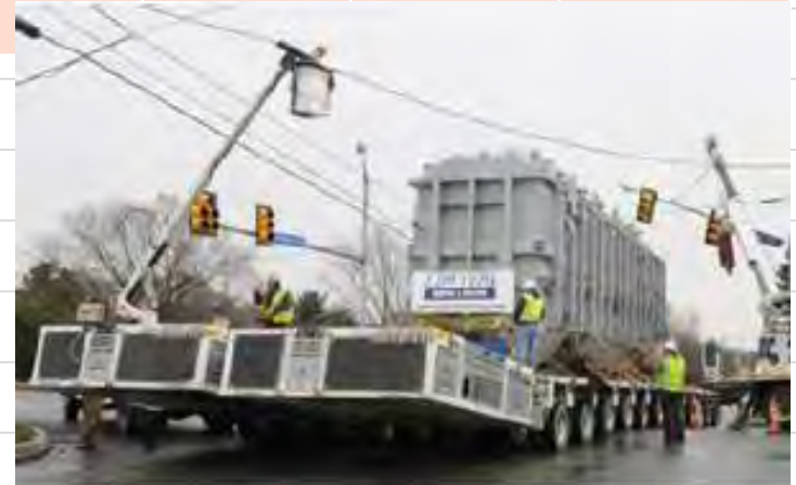
Note: Workers move wires, lights, and poles to transport a 340-ton power transformer, causing hours of traffic delay. Source: Pittsburgh Live News, December 2011.
