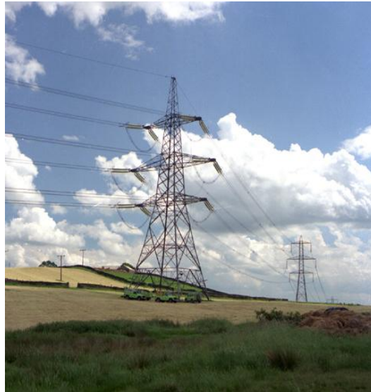
Figure 1 A typical high-voltage transmission line.
